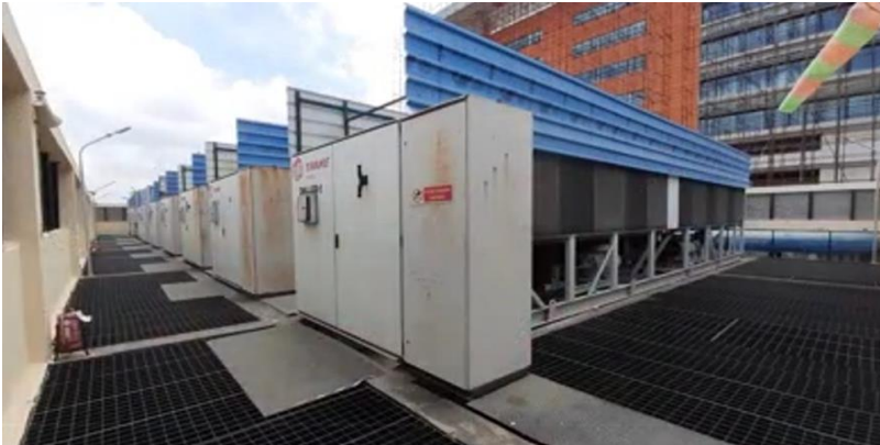
Existing System: Air cooled chiller
