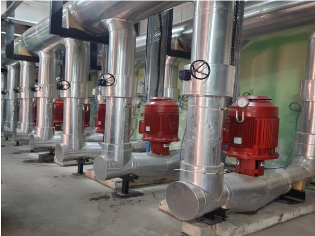
Implemented System: Variable primary flow pump system
