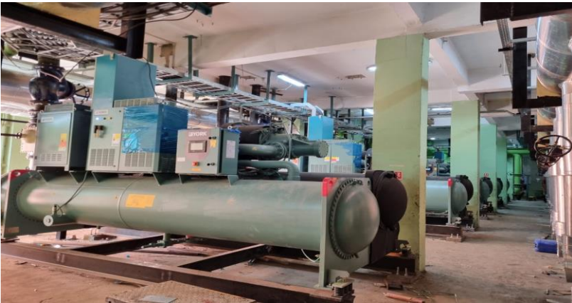
Implemented System: Hybrid Water cooled & Air-cooled chiller
