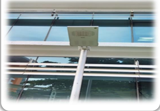
MHL 70W with Solar LED 20W peripheral location
